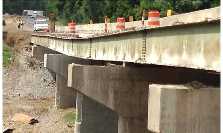
Construction inspections were completed as a part of Primera's work with INDOT's LaPorte District.
